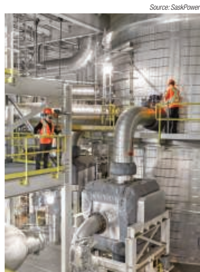
FIGURE 2. A view inside the CCS facility of SaskPower's Boundary Dam Unit 3 in Canada. This plant, with more than one year of operation, is the world's first coal-fired power plant to capture and store the CO 2 from the fluegas
