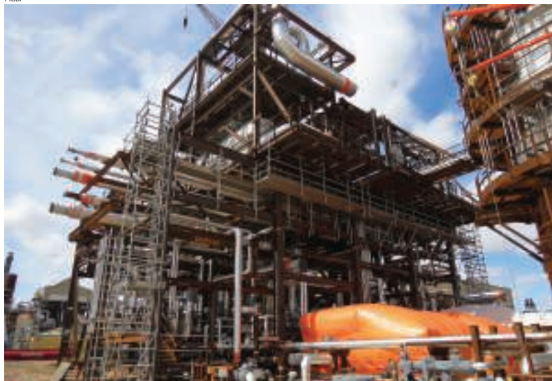
FIGURE 2. On the Shell Quest Carbon Capture and Storage Project in Canada (see also Newsfront on pp. 16–19), Fluor used its 3rd Gen Modular Execution approach to reduce the project's plot space requirements, optimizing process block layouts and consolidating equipment into modules
